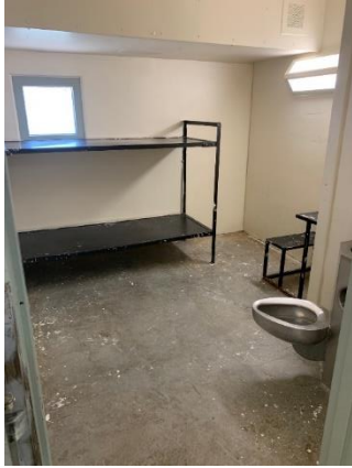
Figure 3. Photograph of a “wet cell” from Coastal Evaluation Center
